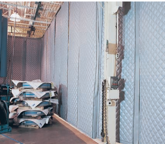
Individual curtains slide along the overhead tracks, making it easy for workers to move stock in and out of the press area.
