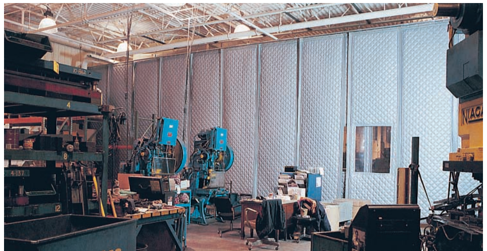
The acoustical curtains block and absorb noise from the presses, reducing noise levels in the plant from 108 dB to about 90 dB.
