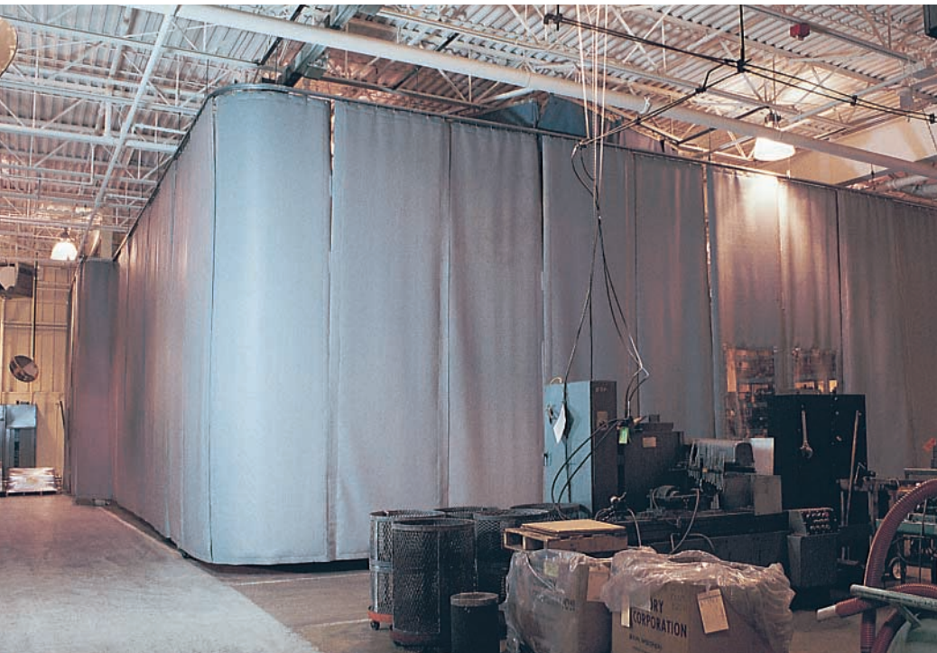
Hayes Industrial Brake met OSHA noise standards by enclosing its punch presses with an L-shaped system of acoustical curtains hung from overhead tracks.
