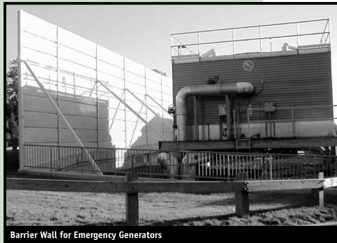
Barrier Wall for Emergency Generators
