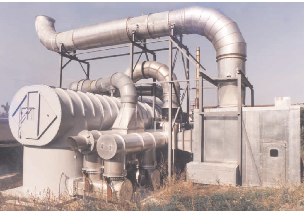
McGill AirSilence supplied a silencer, double-wall elbow, and acoustical enclosure to reduce noise levels at Bradford Industries' facility in Massachusetts.
